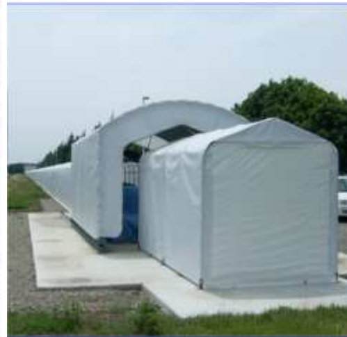
630 m long line for jacketing superconducting cables
